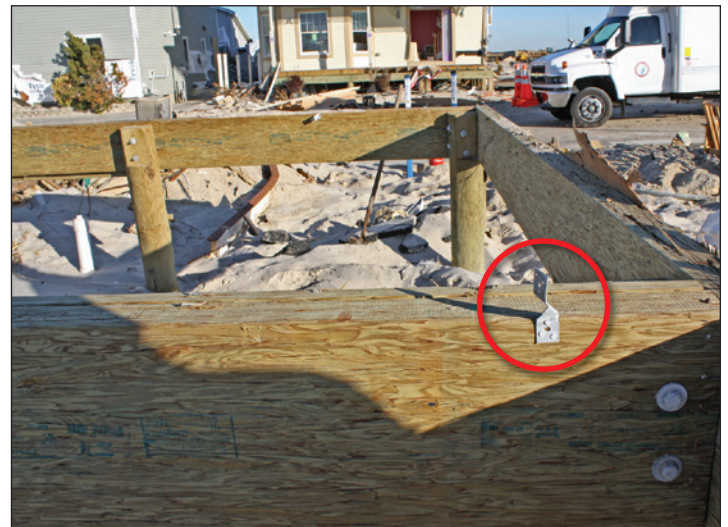
Figure 1: Building with insufficient connectors (red circle) washed off its pile foundation when elevated floor-to-pile connectors failed. Stronger connectors were used on the house in the background (Ortley Beach, NJ).
