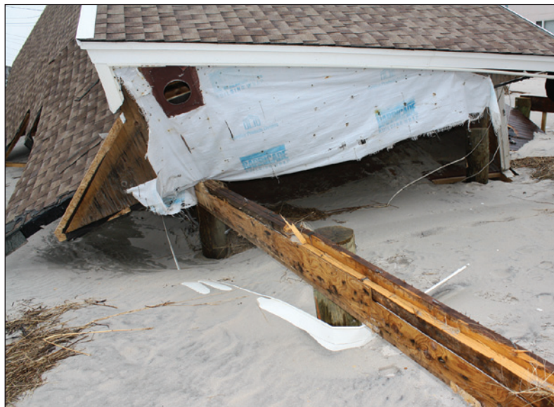
Figure 3: Building with connectors nailed along the grain in the upper edge of the wood beam resulted in the beam splitting (Beach Haven, NJ).
