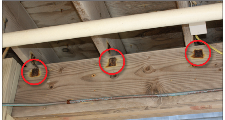
Figure 5. Corroded connectors (red circles) and lack of blocking between joists meant there is no longer a continuous load path providing uplift and shear transfer to foundation piles (Fire Island, NY).
